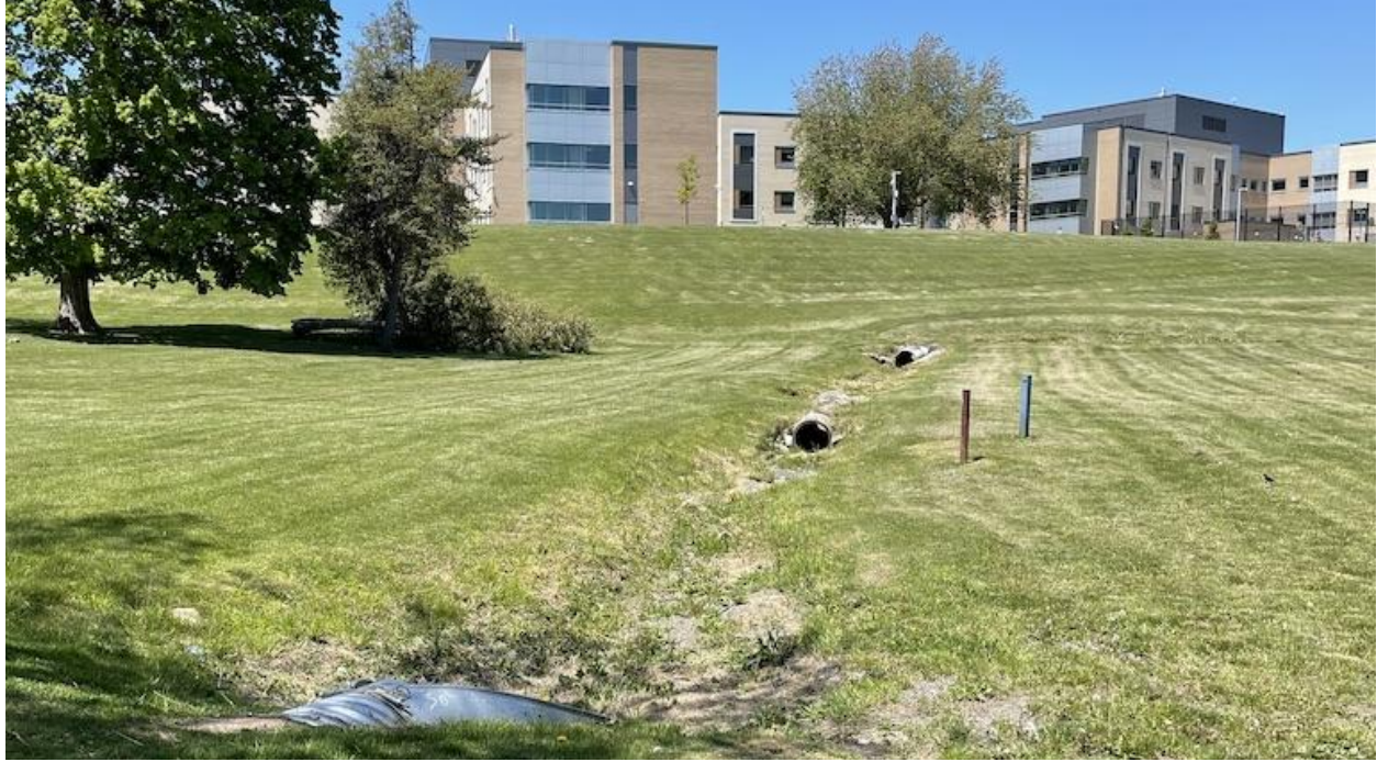
Figure 6. Stormwater Drain Pipe located downhill from Providence Care Hospital and into the swimming area of Hospital Beach.
