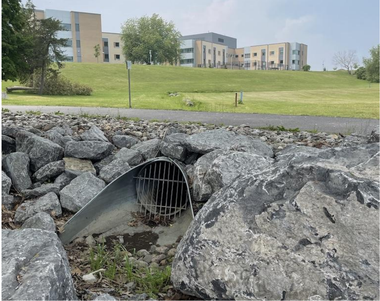
Figure 7. Stormwater Drain Pipe located downhill from Providence Care Hospital flowing directly into the swimming area of Hospital Beach.
